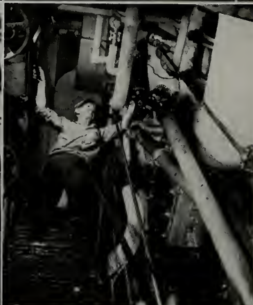
▲ Left: Combustion control panel showing the automatic oil control in the center box while the two side boxes operate the forced drafts; also the steam gauges, water glasses and Pyrometer.
